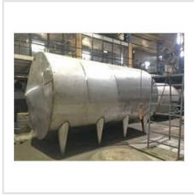
Industrial Milk Storage Tank
