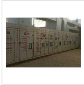
Electric Control Panel
