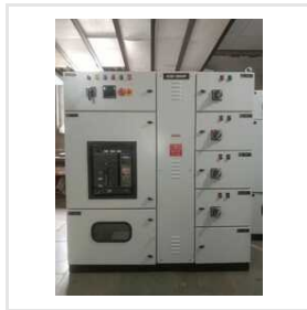
Industrial Acdb Panel
