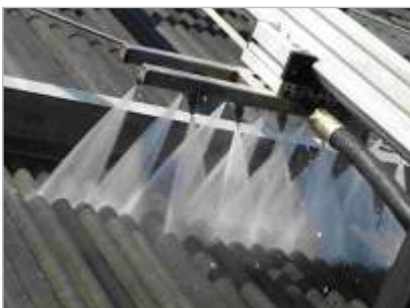
Pump for ACC Fin Tube Cleaning
