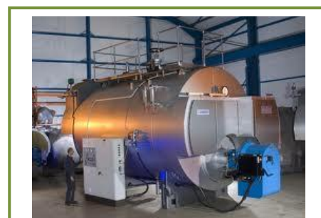
Boiler Pressure Test
