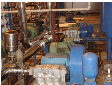
R O pump for Effluent Recycle
