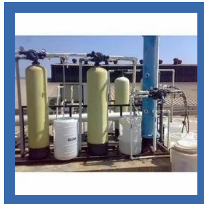
Water Demineralization Plant
