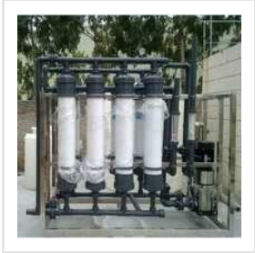
Ultra Filtration Plant
