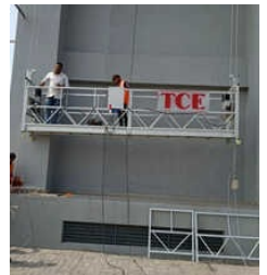
Rental Rope Suspended Platform
