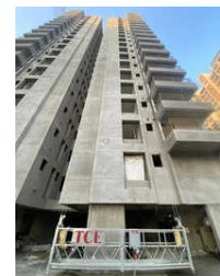
Suspended Hanging Platform
