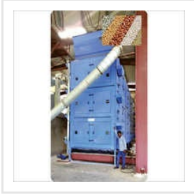
Pulses Drying Plant
