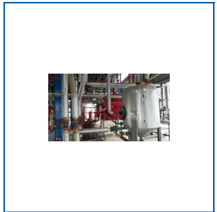
CONTINUOUS PHYSICAL REFINING PLANT
