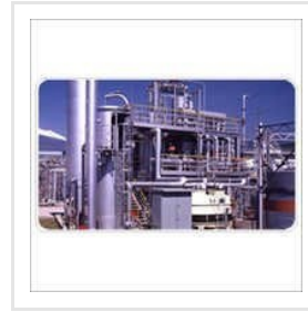
Hydrogen Production Unit
