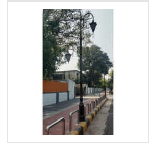
Outdoor Lighting Pole
