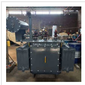
Three Phase HT Power Transformer
