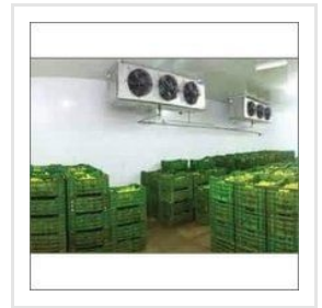
Pre Cooling Chambers
