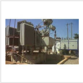
Industrial Transformer Oil Filtration Plant
