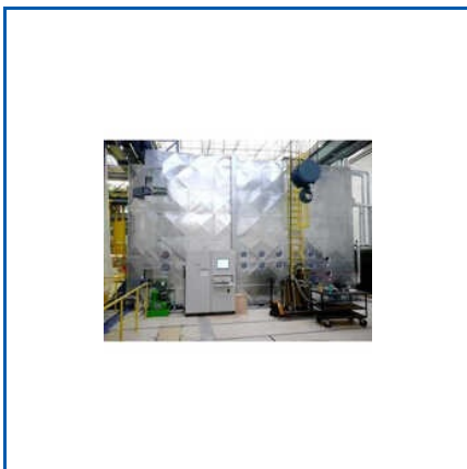
ELECTRIC VAPOUR PHASE DRYING PLANT
