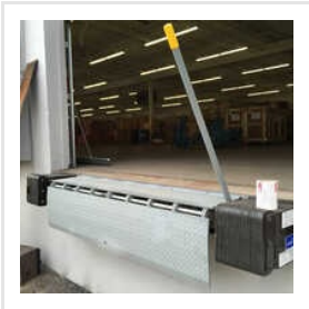
Edge Of Dock Levelers
