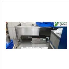
Oil And Grease Trap With Grease Dispenser
