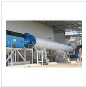
Drum Rotary Dryer (Wooden Fire Base)
