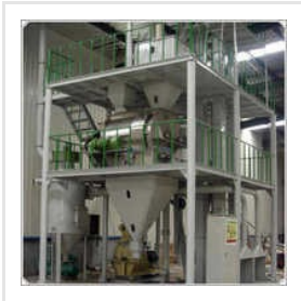
Computerized Cattle Feed Plant
