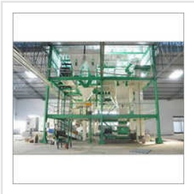
Vertical Feed Plant
