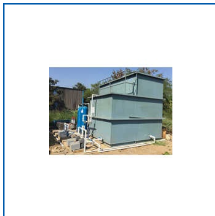
PACKAGED SEWAGE TREATMENT PLANT
