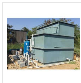
Packaged Sewage Treatment Plant
