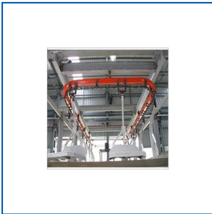
OVERHEAD CONVEYOR SYSTEM
