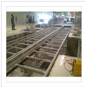
125 Mtr Final Assembly Line Conveyor
