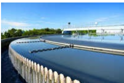
Effluent Treatment Plant
