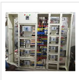
LT Distribution Panel
