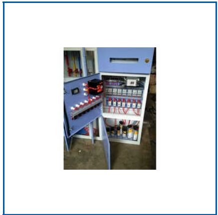
APFC POWER CONTROL
