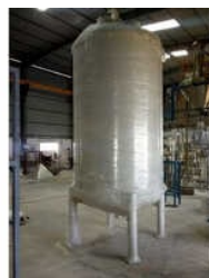
Chemical Process Tank
