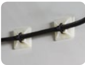
Inside the control panel
