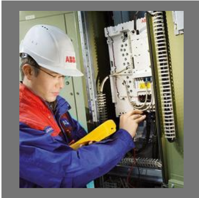
AC Drives Service Center
